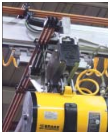
Electric supply using Insul-8
